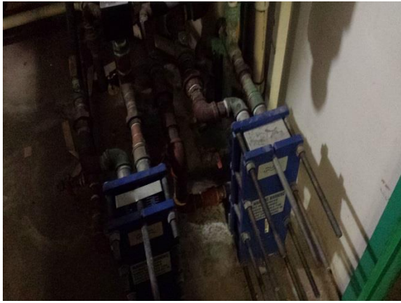
Limited Access to key pieces of equipment made it difficult to maintain the original system.
