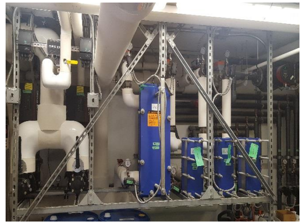
New installation is easily accessible for inspection and ongoing maintenance. Raising the equipment also provides valuable floor space within a limited footprint.
