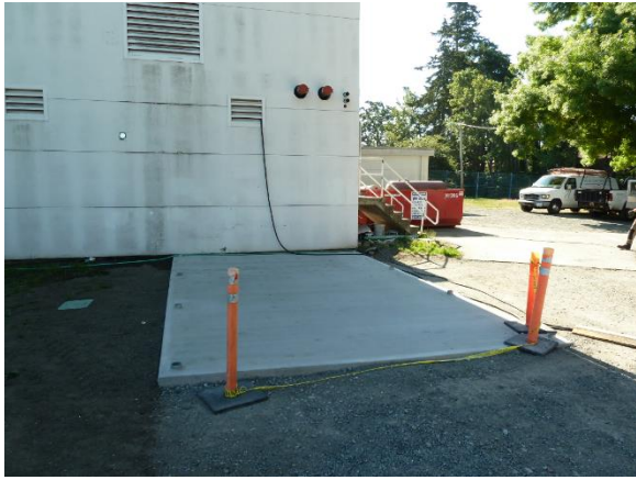
Location prepared for new ASHP includes plumbing and electrical ‘rough-in’ as well as seismically rated concrete pad.
