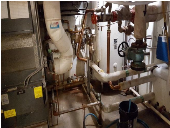
Original boiler plant was cluttered and inaccessible
