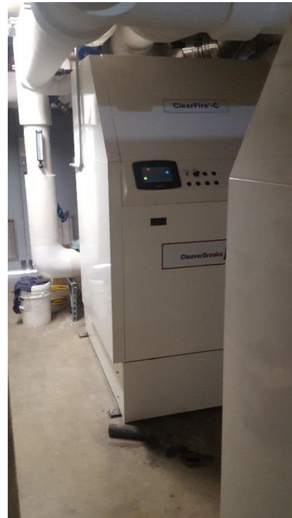
New plant is fully automated and more efficient
