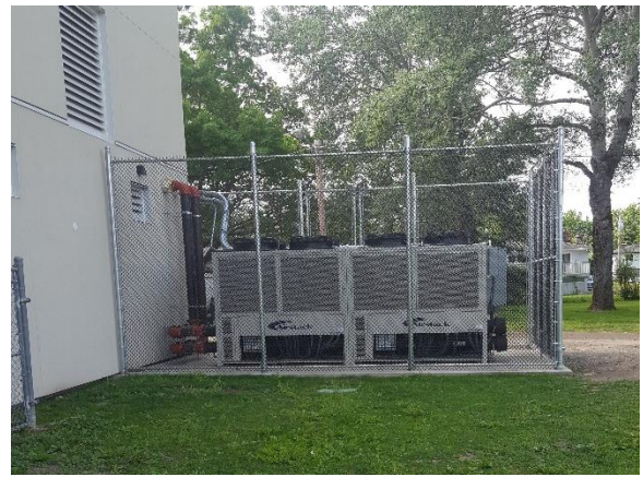
New ASHP secured with unclimbable chainlink fencing.
