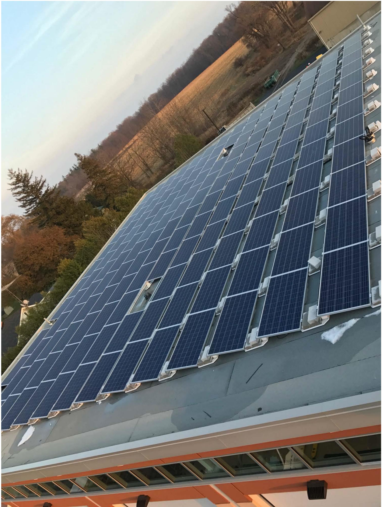
Coldstream Fire Station – Solar Panels Photo Credit: Jamie Smith Photography
