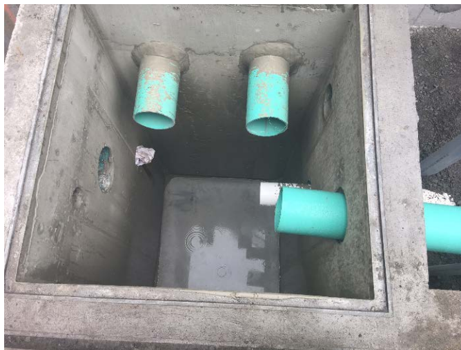
Photo 2: Air extraction piping at dedicated sump for the sub-slab gas venting system
