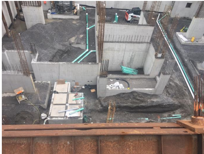
Photo 1: Layout of solid header pipes (tourquise colour) for sub-slab gas venting system
