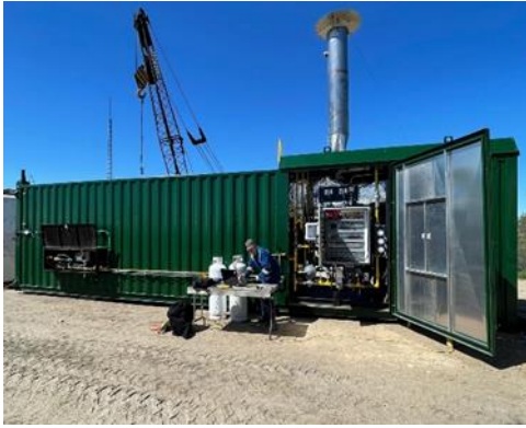
Completed Gasifier Unit System – 2021
