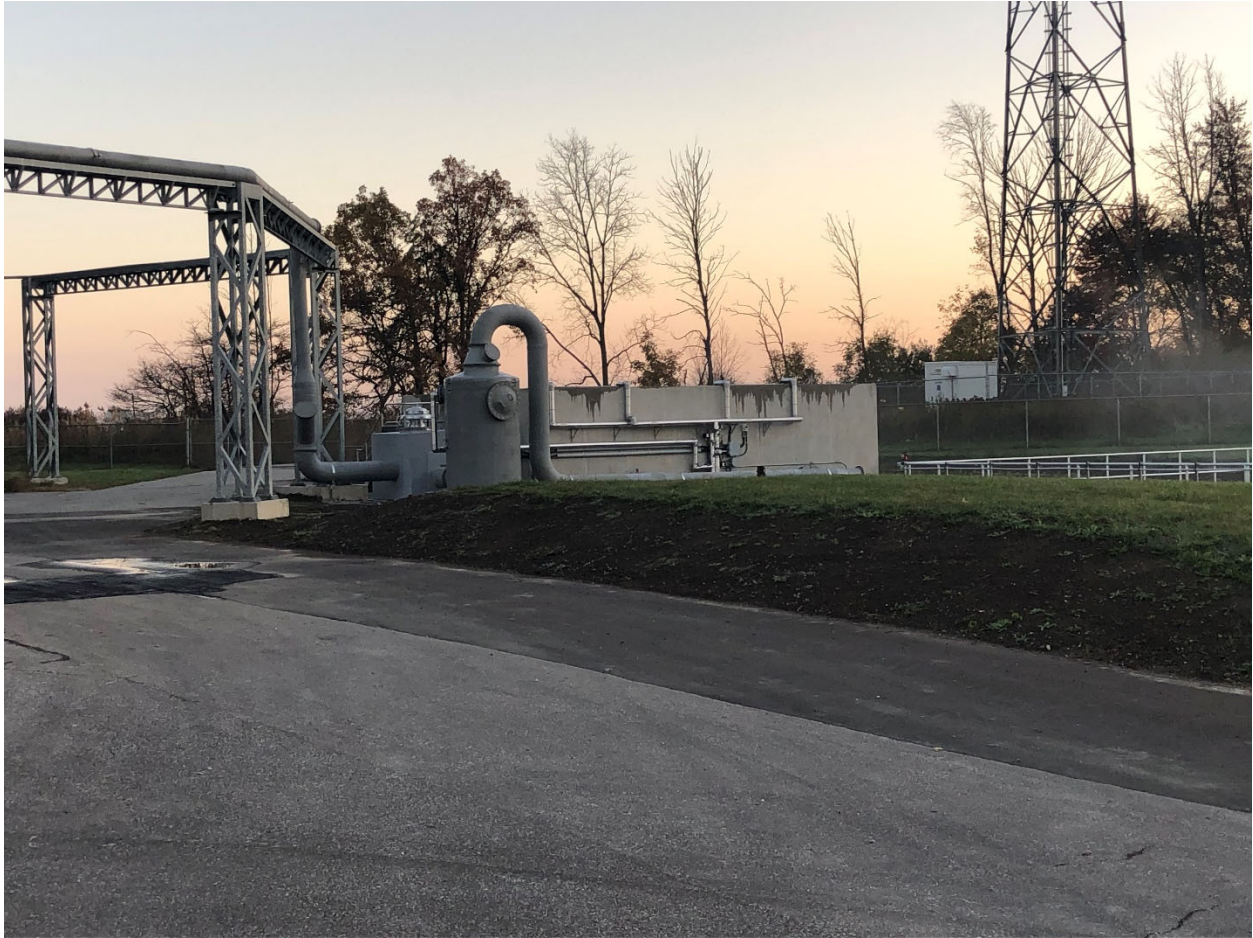
PICTURE OF THE COMPLETED ODOUR CONTROL UNIT, PIPE RACK, HUMIDIFIER AND BLOWER
