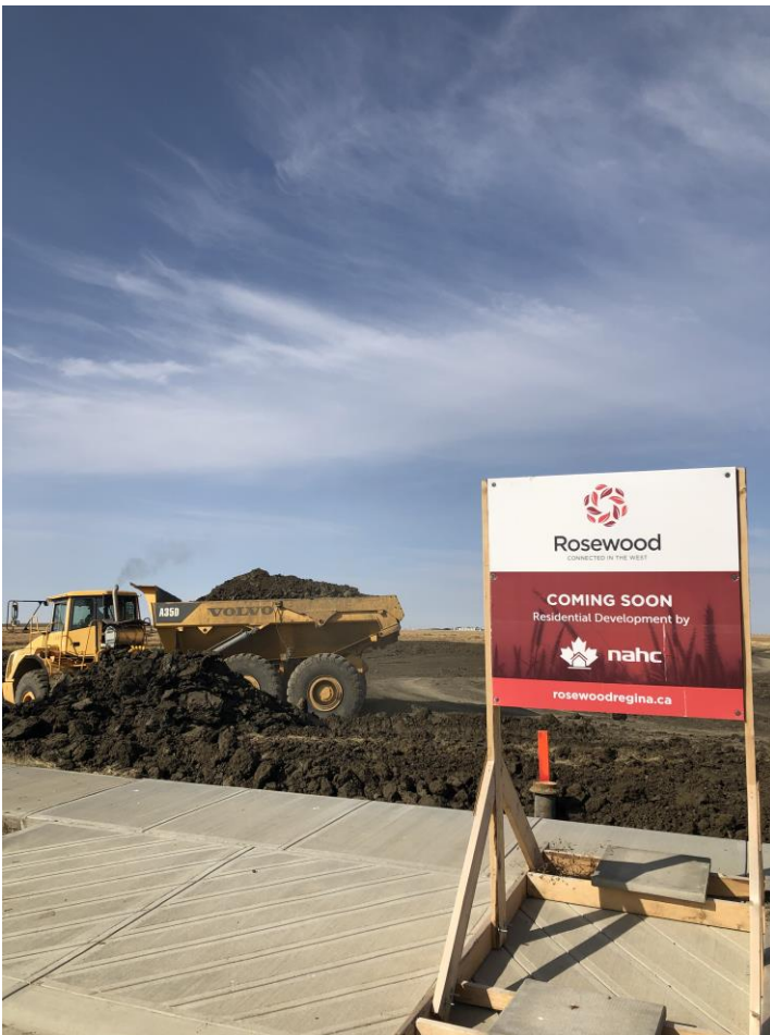
Before Photo – View of Plainview Townhomes site facing west in Regina, SK. Located at 1420 N Silverleaf Blvd. Photo taken prior to project development; subdivision parcel grading work being completed by Rosewood subdivision developer.
